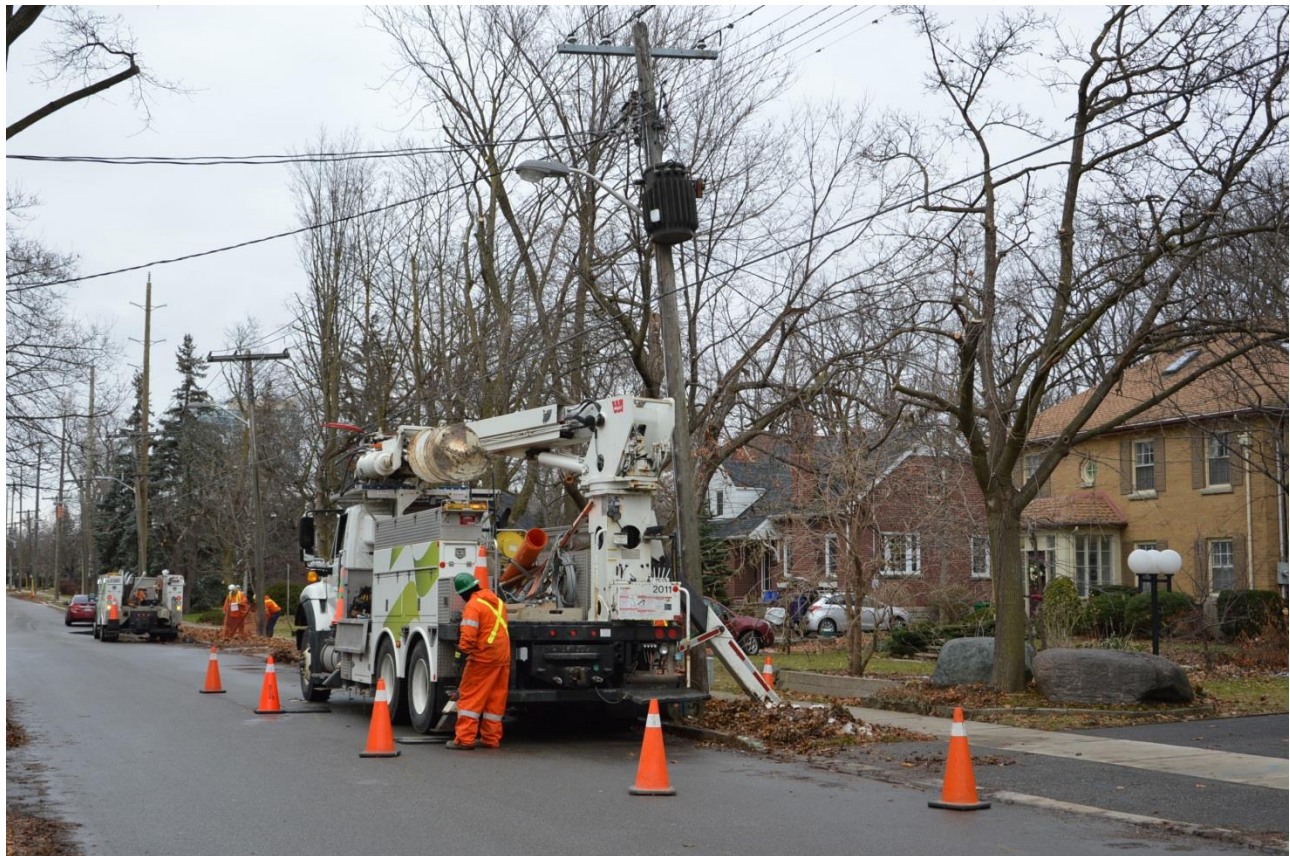
Alectra crews working to upgrade infrastructure for homes and businesses in Brampton.
